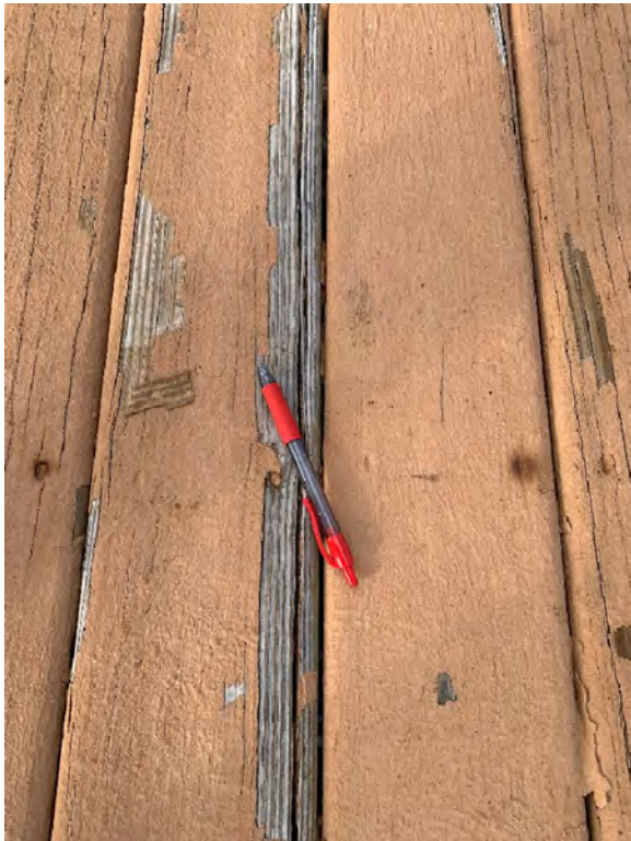
Dry-rotting, splintering and splitting deckboards
