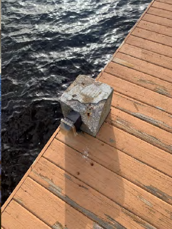
Spalling pile previously repaired
