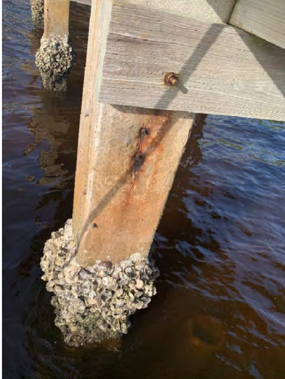
Rust-bleeding and cracked pile
