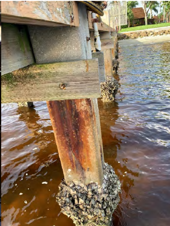
Severely cracking and rust-bleeding pile
