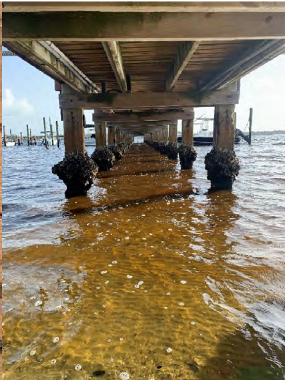
Cracked piles, framing showing signs of splitting, mildewing
