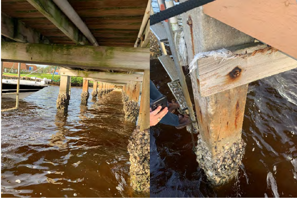
Splitting framing members, mildewing wood Cracked pile, rotting pile cap framing
