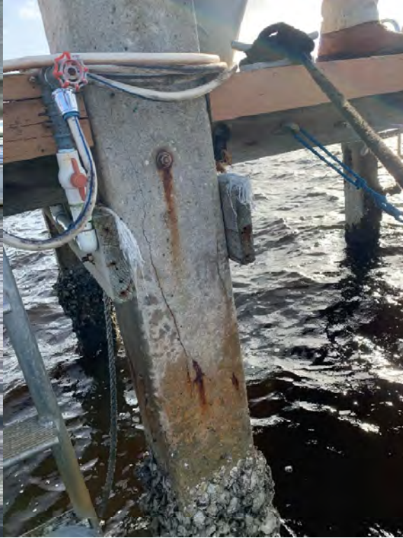
Rust-bleeding and severely cracking pile
