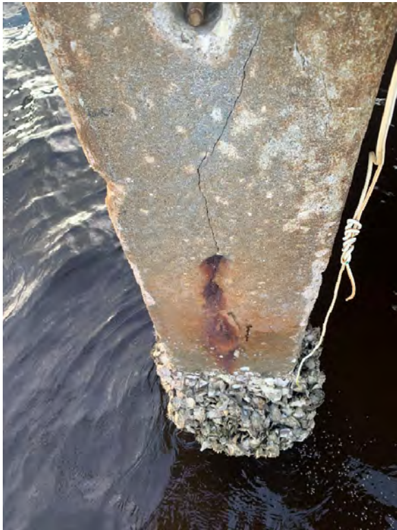
Severely cracking pile
